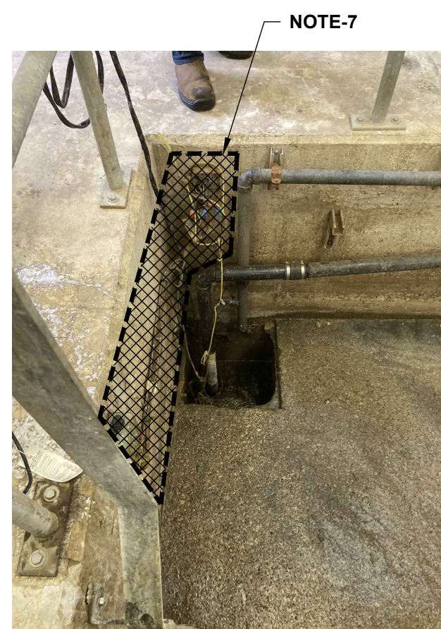
FIG.9 - SUMP PUMP BLOWER ROOM
