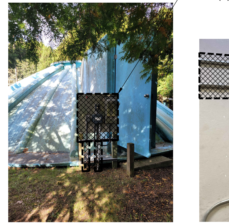
FIG.3 - CLARIFIER LOCAL CONTROL PANEL
