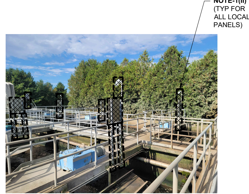
FIG.2 - AERATOR LOCAL CONTROL PANELS
